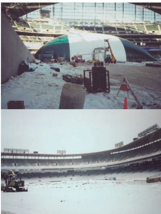
One of Bossard’s most challenging stadium projects was Miller Park in Milwaukee. With over a foot of snow on the field and frozen turf, specially designed heating tents had to be brought in to house the 2-million BTU heaters for 12 days to install the irrigation system and the turf.
